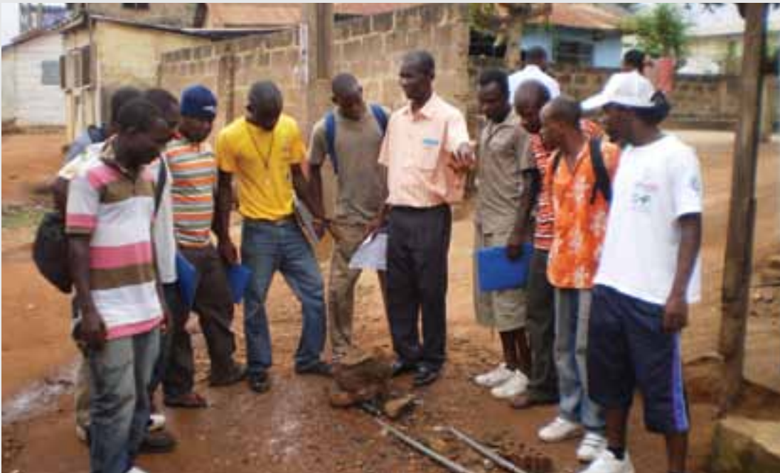
Ghana: Community plumbers undergo a hands-on training.
